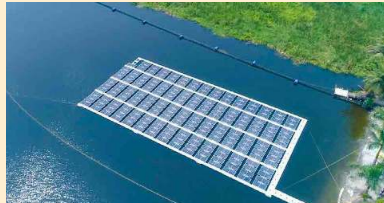
Micro-grid: 100 kWp Floating Solar Plant commissioning (along with Floating Solar & Battery) work in progress at Chakmir 132/33 kV S/S
