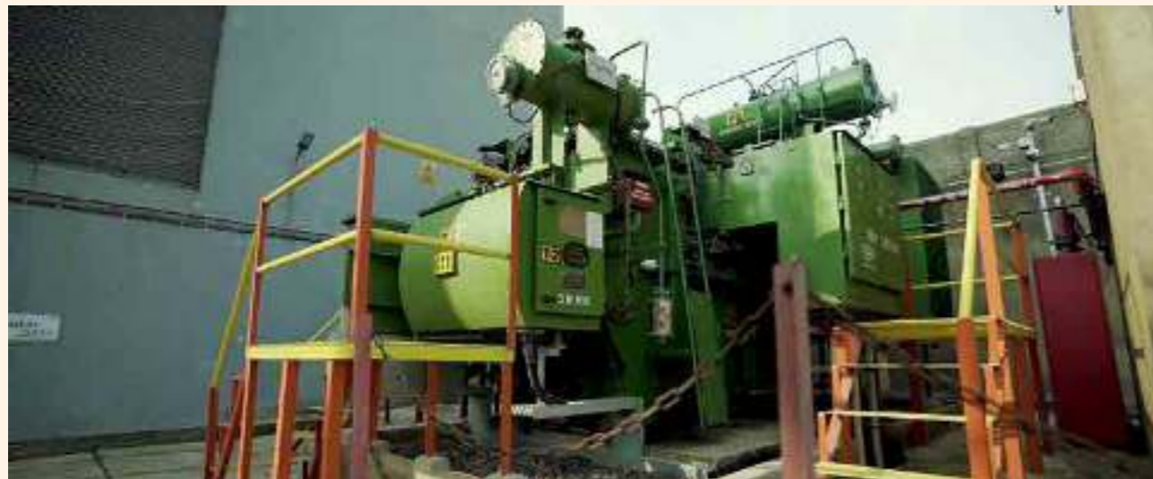
Ester oil filled power transformer
