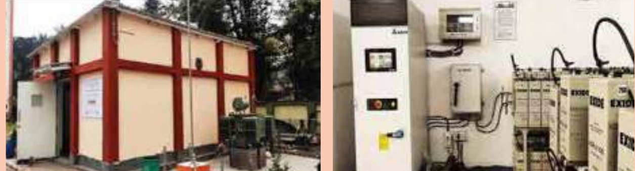
Grid Connected 315 KWH BESS Installed at East Calcutta Substation
